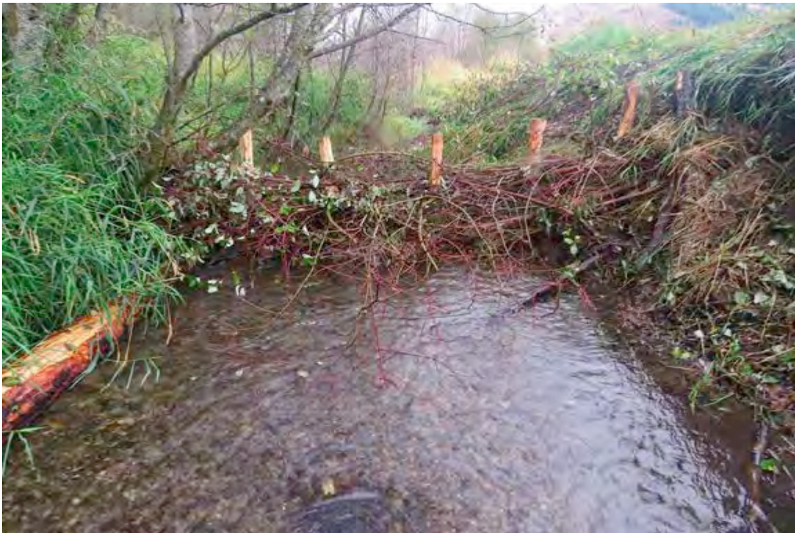
Figure 80: Pilings woven with live red oyster dogwood, some of which was planted directly into the exposed bank to facilitate resprouting
