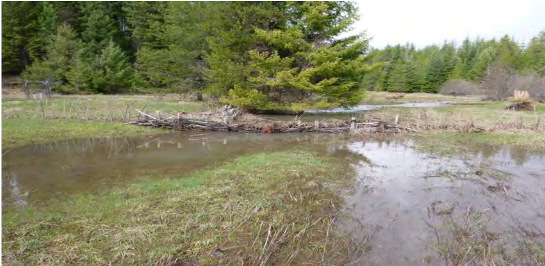
Figure 58. BDAs after peak flow constructed with posts driven into the streambed and woven with wicker weaves.
