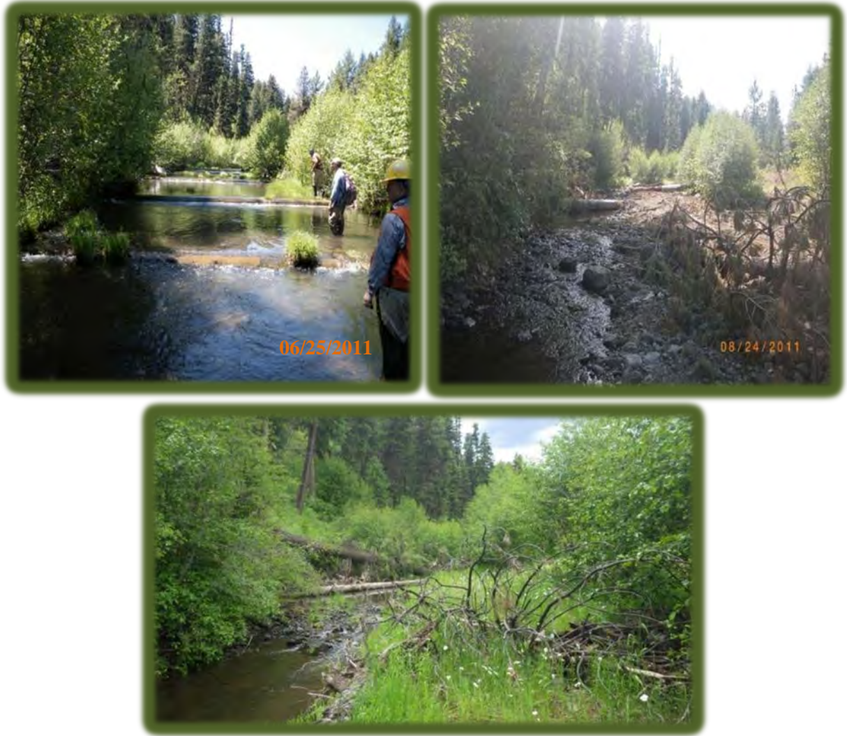
Figure 49: Log Weir Removal from Reach 4 of Camp Creek before (top left), immediately after (top right), and 3 years later (bottom)
